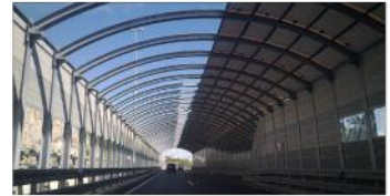
A sound barrier tunnel on the Croatian A7 motorway near Rijeka. The motorway is approximately 130 feet away from residential area, most notably a 26 story building. Source: Croatian Motorway Authority
