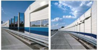
Steel and glass noise barrier along a highway in Vienna, Austria. Geometry used to break the noise path from the source to the receiver is critical. Optimal effects are obtained if the screen is placed as close as possible to the highway or next to the receiver. Source: "Noise Barrier Design" Hans Bendtsen
